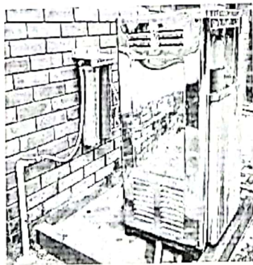
Fig:2. Drinking water cooler
